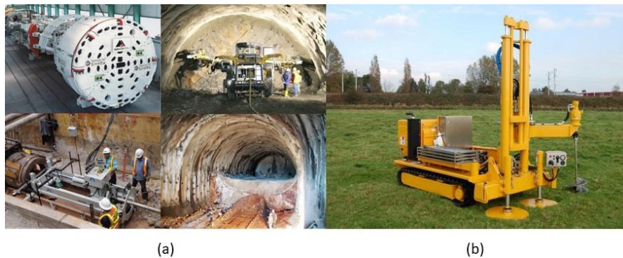
Figure 1.1: Illustration of various methods of geotechnical penetration : (a) Tunnel boring machines (TBMs), drill and blast, shielded excavation machines (SEMs), and micro tunnel boring machines (MTBMs). The four methods are illustrated in clockwise order from the top left corner of the figure. The images used in the illustration are obtained from sources such as Heitkampt-swiss.ch, Akkerman.com, and a publication by Hoek et al. in 2007. ; (b) Cone Penetration Test(CPT)- Image from Structville
