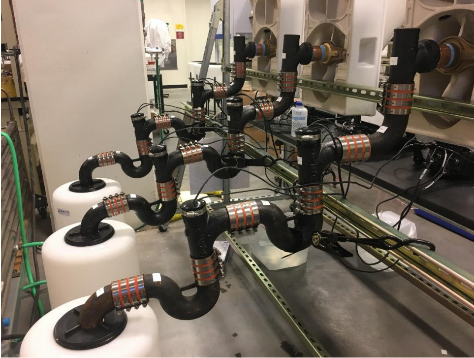
Figure 3-S11. Back of urinal testbed. Two-inch cast iron pipe is used to convey the urine from the urinals to the storage tanks. Two P-traps were used to hold pH and conductivity sensors in urine solution.
