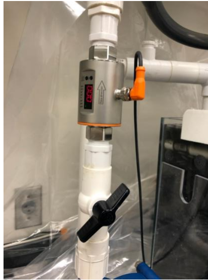
Figure 16. Ball Valve controlling the recirculation flow rate.
