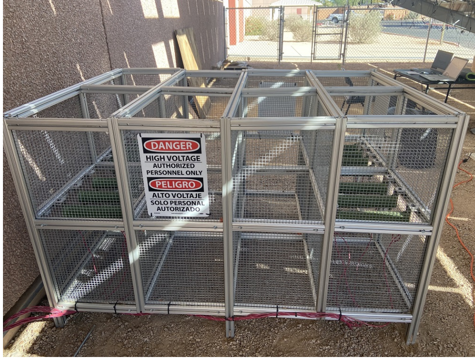
Figure A.5: A load bank consisting of multiple resistors to collect data in real time. There are 7 resistors. 4 of these resistors are always on and the remaining 3 are turned on depending on the time of the day.
