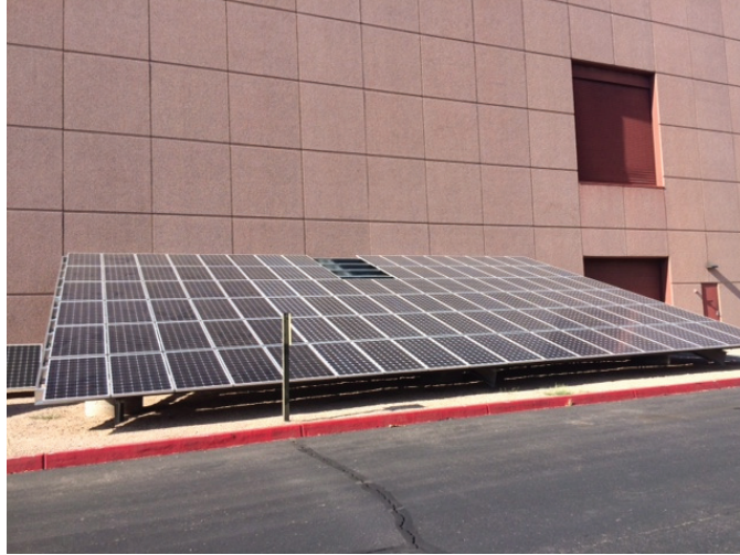
Figure 1.2: The SenSIP Solar Monitoring Facility at the ASU Research Park.
