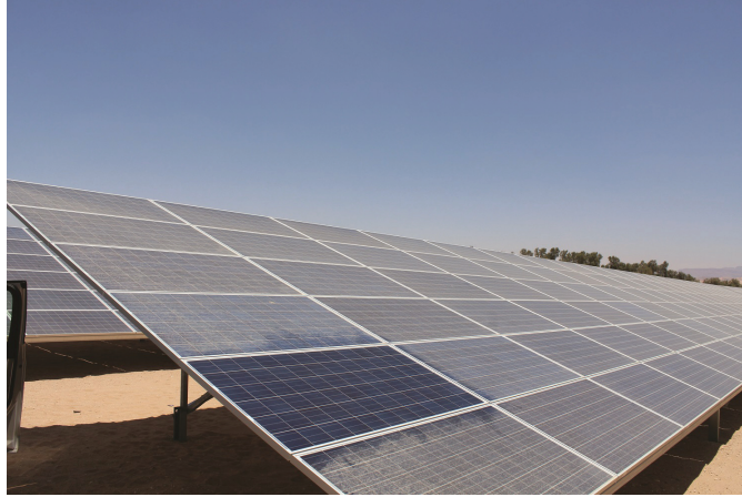
Figure 4.4: Example of a Soiled Solar Panel.
