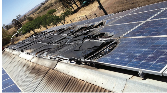
Figure 4.6: Example of Damage from an Arc Fault.
