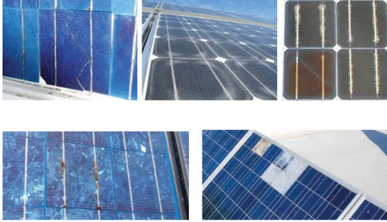
Figure 4.5: Example of a Degraded Solar Panel.
