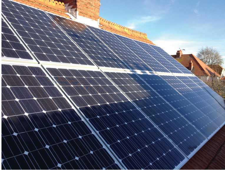
Figure 4.7: Example of a Partially Shaded Solar Panel Array.
