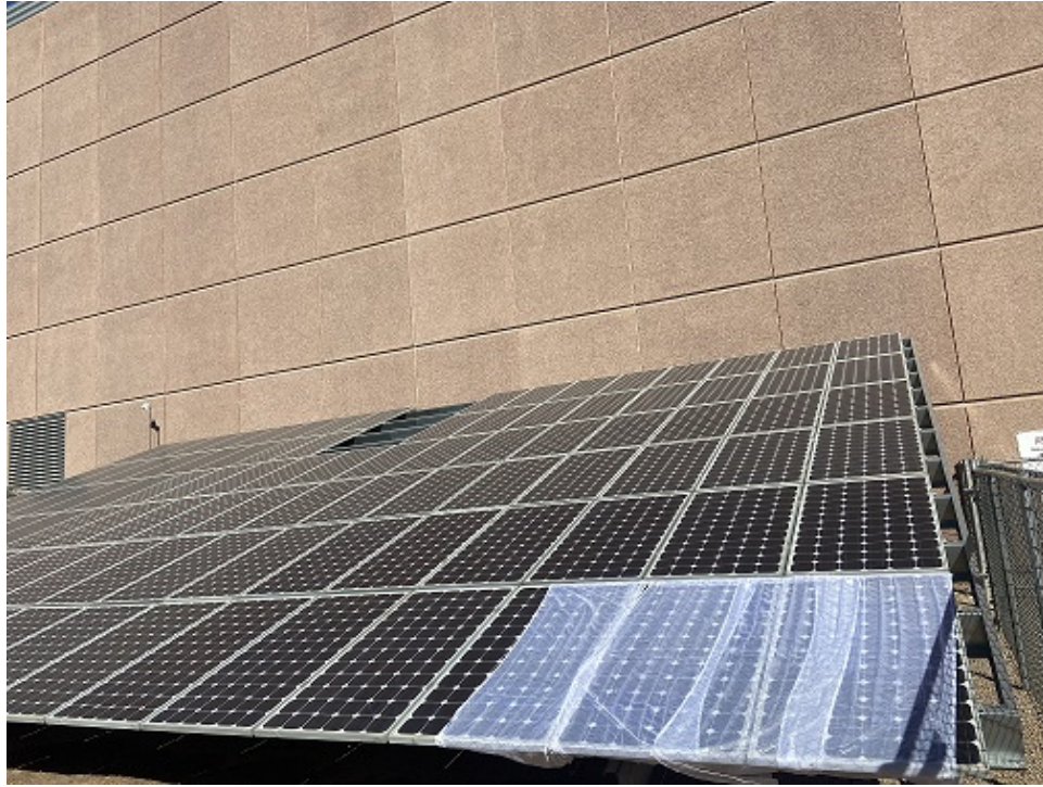
Figure 4.16: An Example of a Simulated Shaded Module at ASU Research Park. This Corresponds to 25% Shading.
