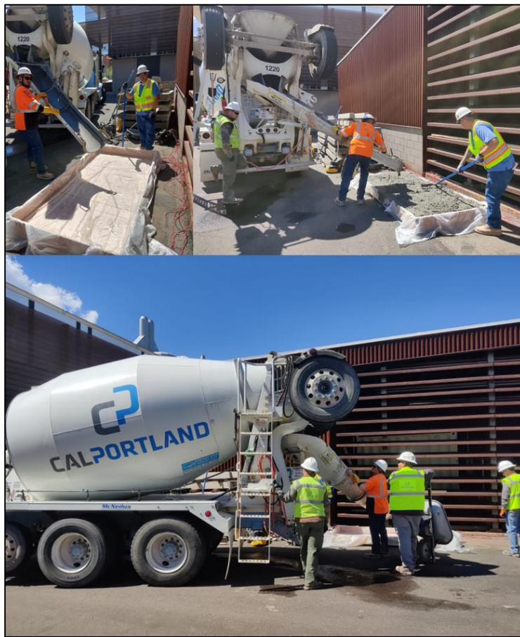
Figure 13: 3.3.3.4 Pictures taken during the casting of the slab with SUNDT workers and CalPortland truck.
