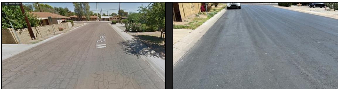
Figure 7-16: Pavement Condition Before and After Thin Overlay on Rose Ln between Black Canyon Frwy (I-17) and 23 rd Ave
