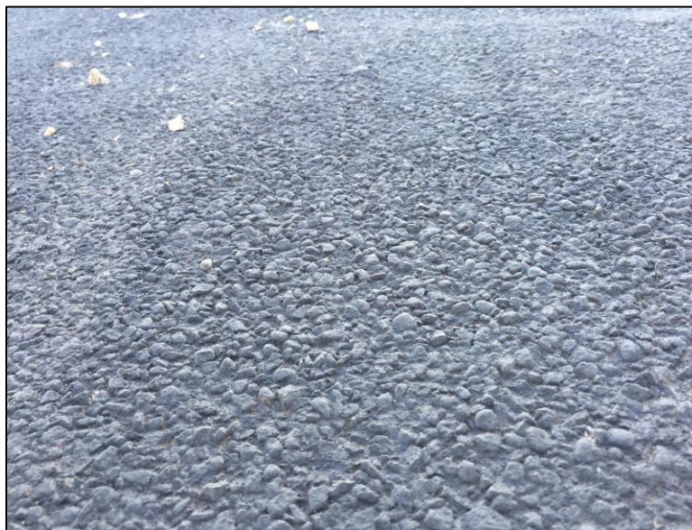
Figure 7-8: Low Volume FAST Capped with a Single Coating of Liquid Road Application
