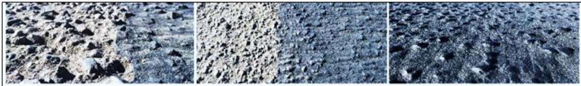
Figure 6-5: Pavement Surface Before and After the First Coat of Seal Coat Application (Left and Center Images) and the Final Surface After the Double Seal Coat (Right Image)
