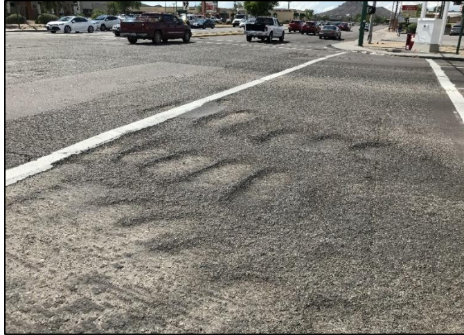
Figure 7-17: Raveling at Intersection
