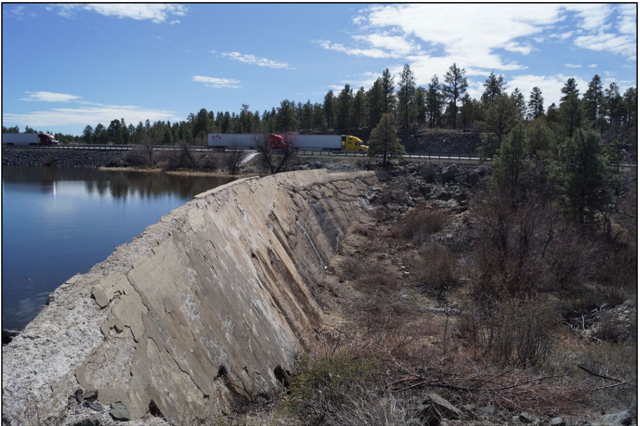
Figure 9. Williams Dam in 2020. The masonry dam is in general poor condition today and actively weeps water through the face of the dam. Daniel Milowski, Williams Dam, 2020. Author's personal collection, Tempe, AZ.
