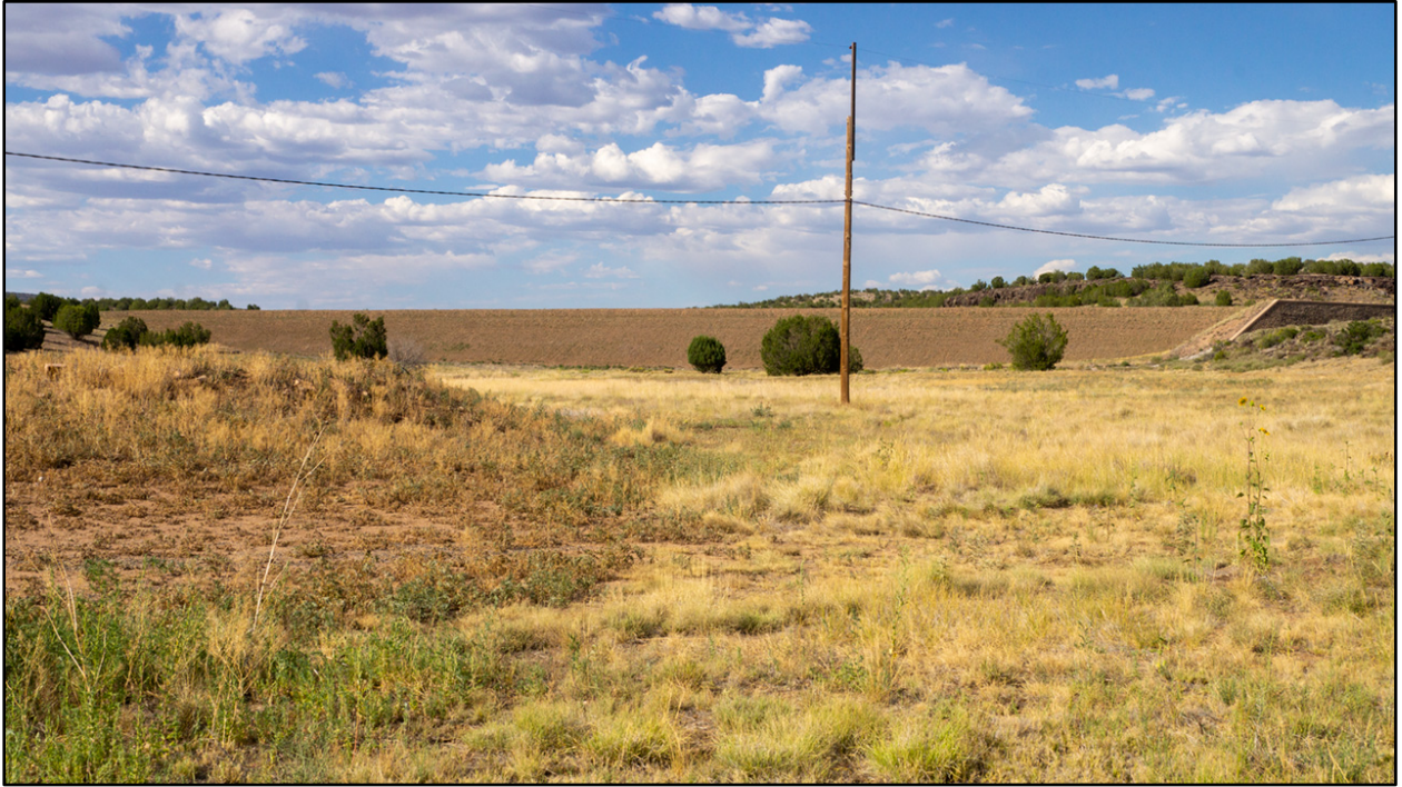
Figure 11. Canyon Mouth Dam in 2020. The dam formerly completely impounded the Big Chino Wash south of Seligman. Today the reservoir is dry. However, deep wells were sunk south of the dam into the Big Chino Aquifer to supply water to Seligman. Photograph: Daniel Milowski, Canyon Mouth Dam, 2020. Author's personal collection, Tempe, AZ.
