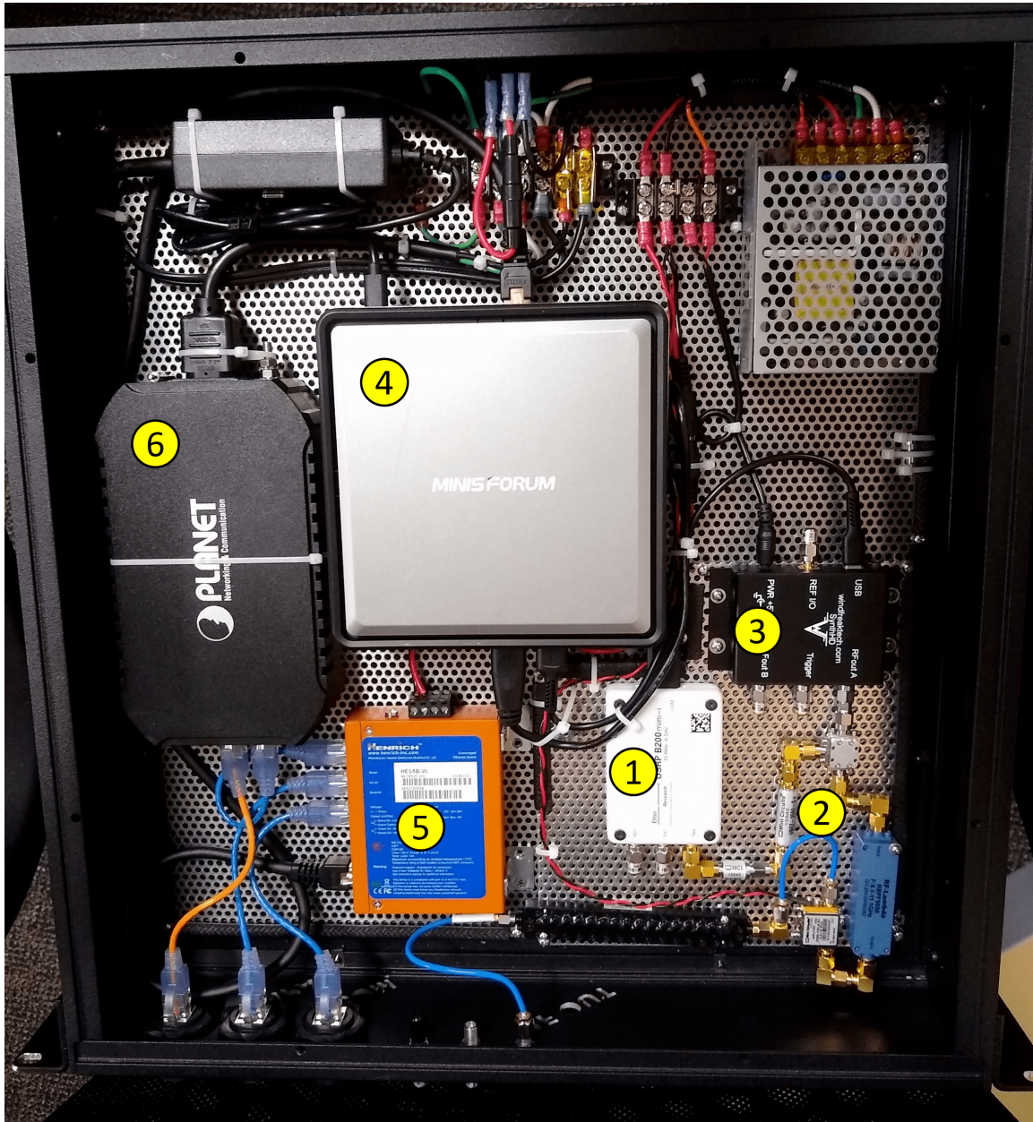
Figure 11: A photo of the components inside System-X's electronics enclosure. Key components are numbered: (1) Ettus B205mini-i SDR (2) X-band upconverter/RFFE (3) Windfreak SynthHD synthesizer (4) Minisforum HM50 (5) Ethernet switch (6) PoE supply.
