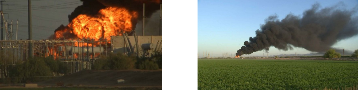
Figure 1. Transformer fire at Salt River Project’s Rudd substation in Avondale, AZ
