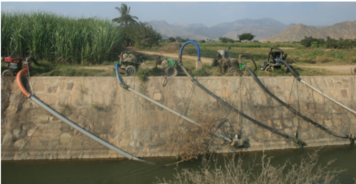
Figure 8. Headenders' Pumps in the Taymi Canal
