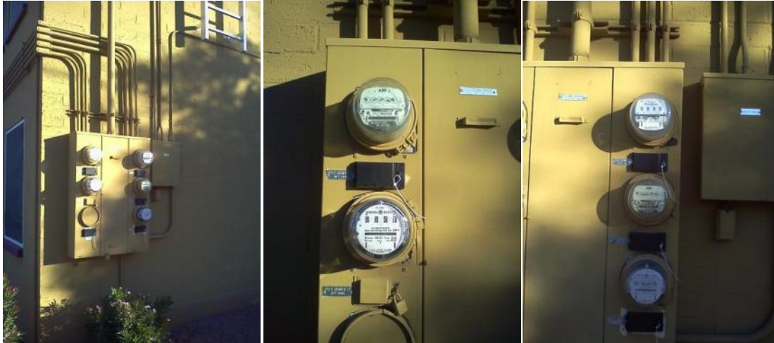
Figure 9. Dashboard selected site electric meter sub-panels close-up
