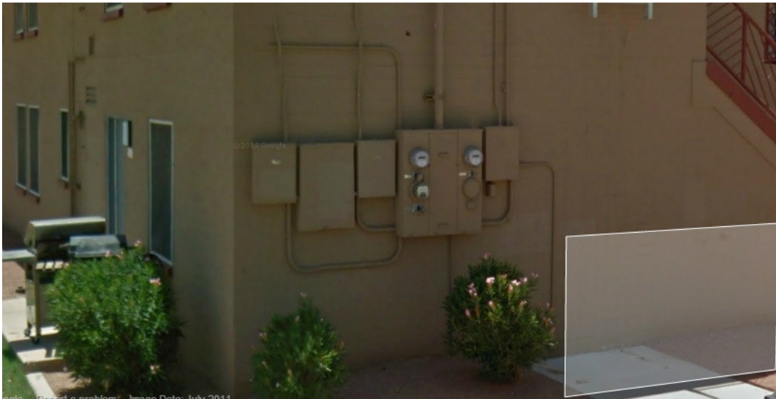
Figure 12. Individually metered apartments, sub-panels outside the unit blocks
