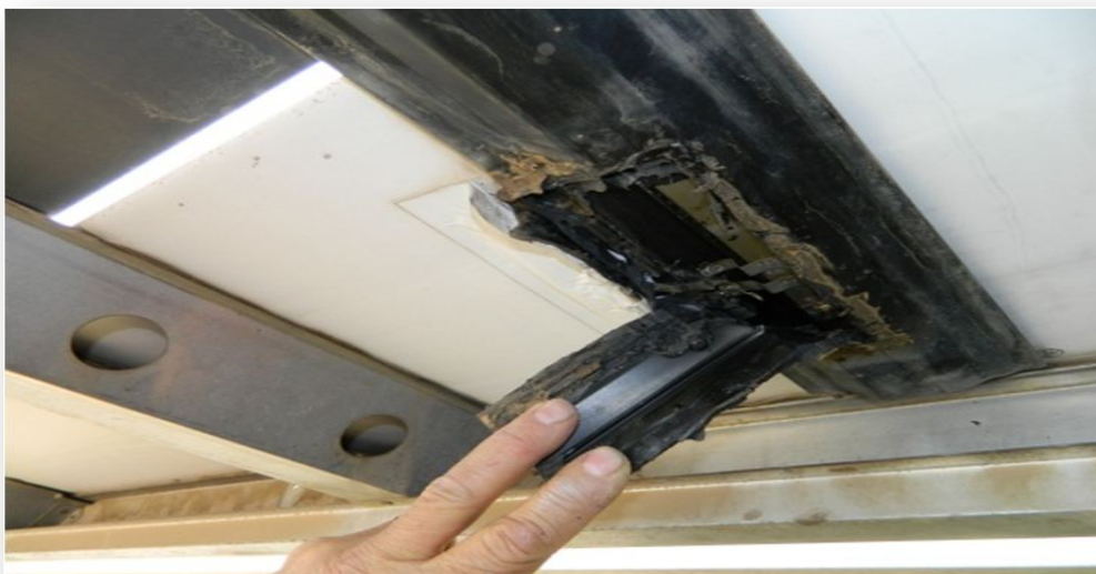
Figure 10 Failed Busbar Seal
