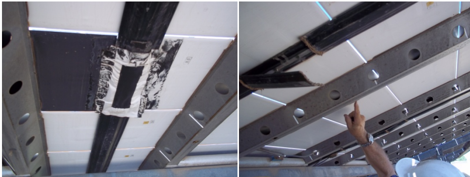
Figure 36- Examples of Busbar Seal Failure
