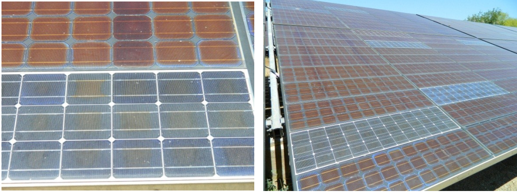
Figure 4.23 Left: Original module on top, replaced module at bottom. Right: Panel group with multiple replacement modules.
