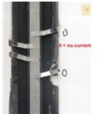
Figure 4.19 Bus bar and panel pre-assembly error
