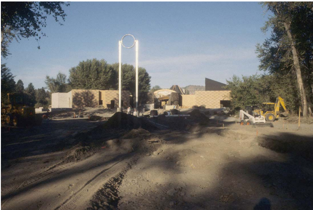
Figure 6.19. East stanchion with building under construction. Courtesy of Stastny Brun Architects from the Stastny and Burke project archives.
