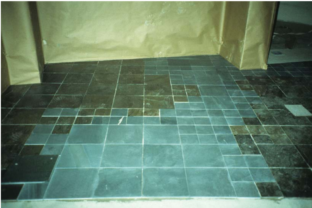
Figure 5.7. Slate tile “stream” in lobby. Courtesy of Stastny Brun Architects from the Stastny and Burke project archives.
