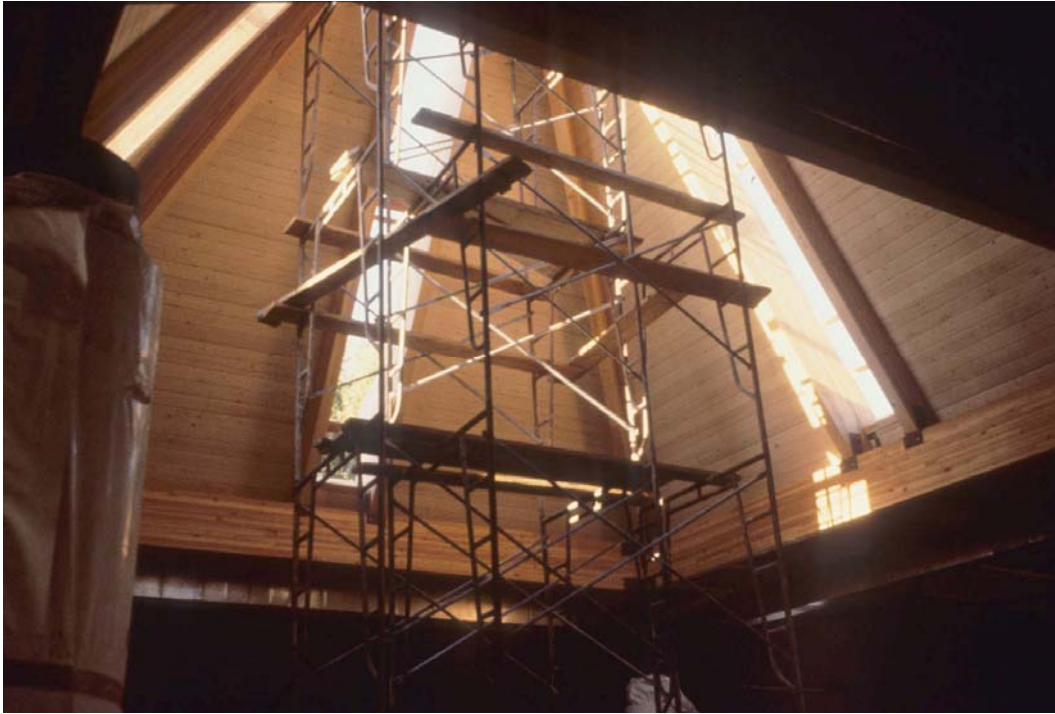
Figure 5.13. Pyramidal ceiling of changing exhibits gallery under construction. Courtesy of Stastny Brun Architects from the Stastny and Burke project archives.
