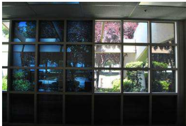
Figure 2: Photochromic glass adjacent to static glazing.
