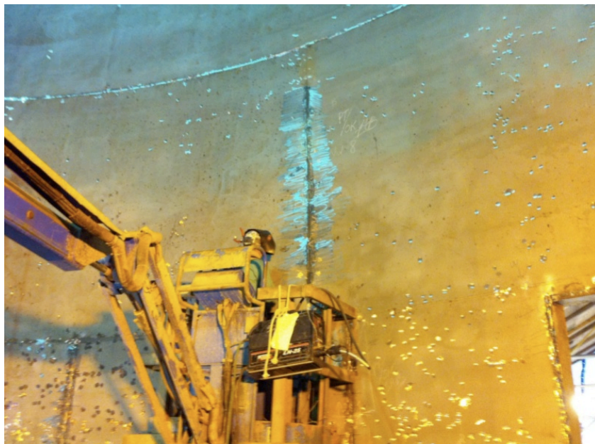
Figure 2.1 Image of Pitting and Stress Corrosion Cracking
