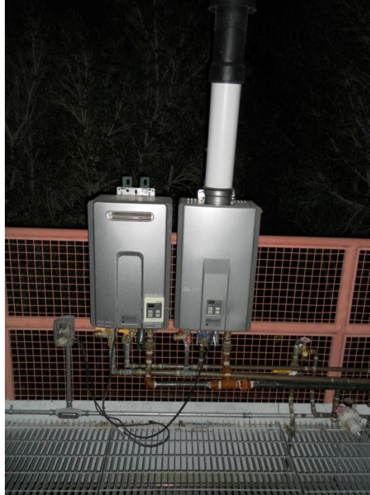
Figure 10. Rinnai Tankless water heaters plumbed in parallel
