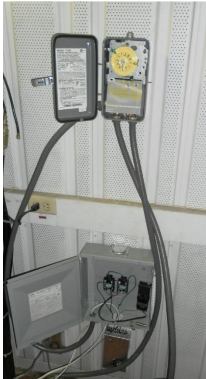
Figure 20. Collector array fluid controller
