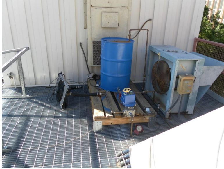
Figure 16. Storage tank, heat dump, and flow control valve
