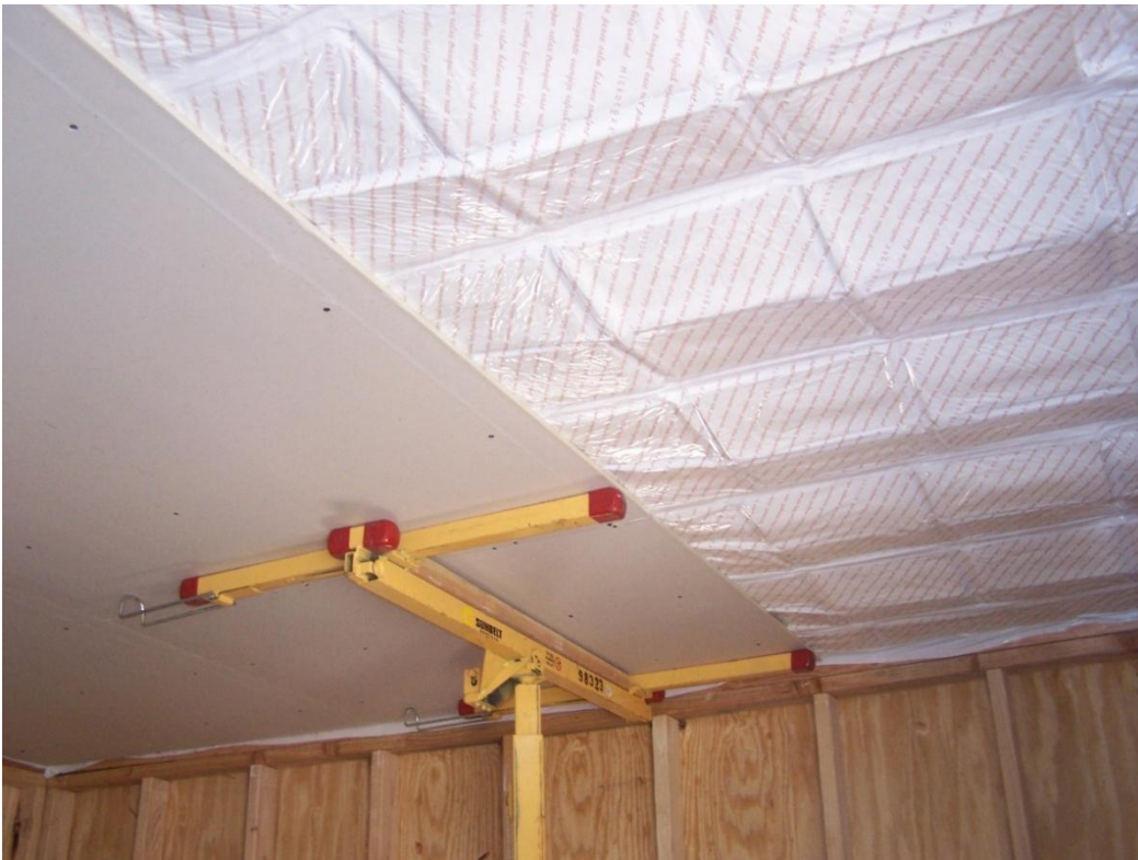
Figure 2.9 Installed BioPCM Mat in the Ceiling
