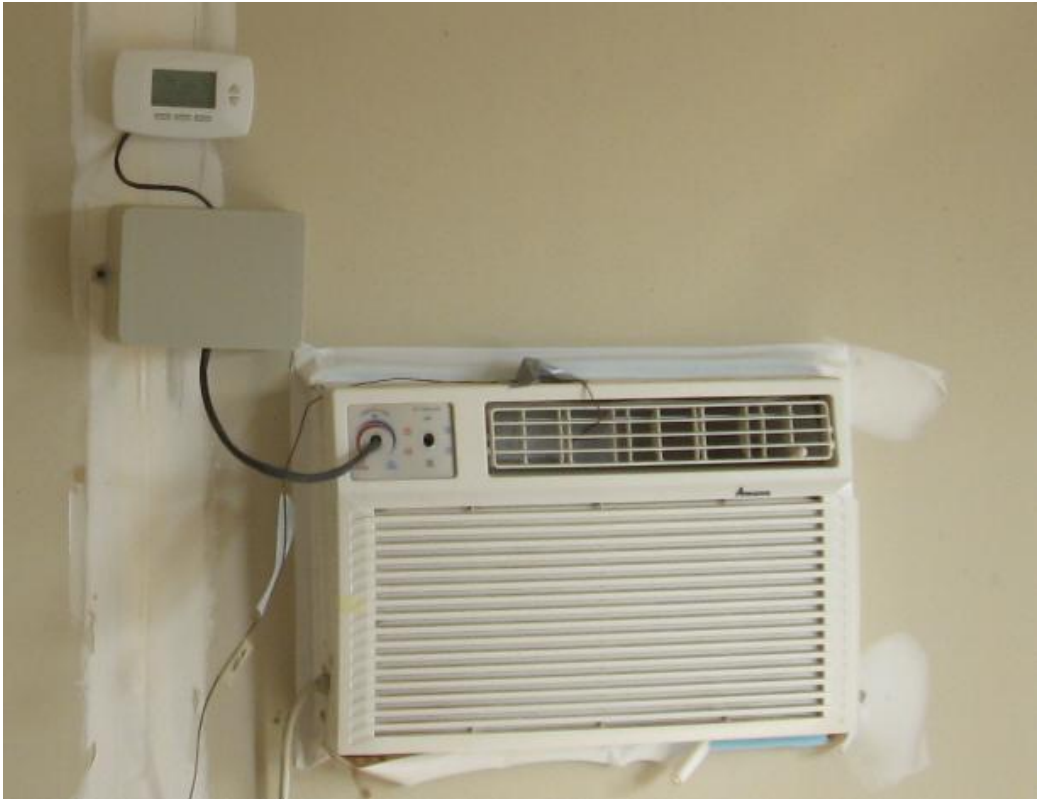
Figure 2.5 Heat Pump and Thermostats used in the Shed
