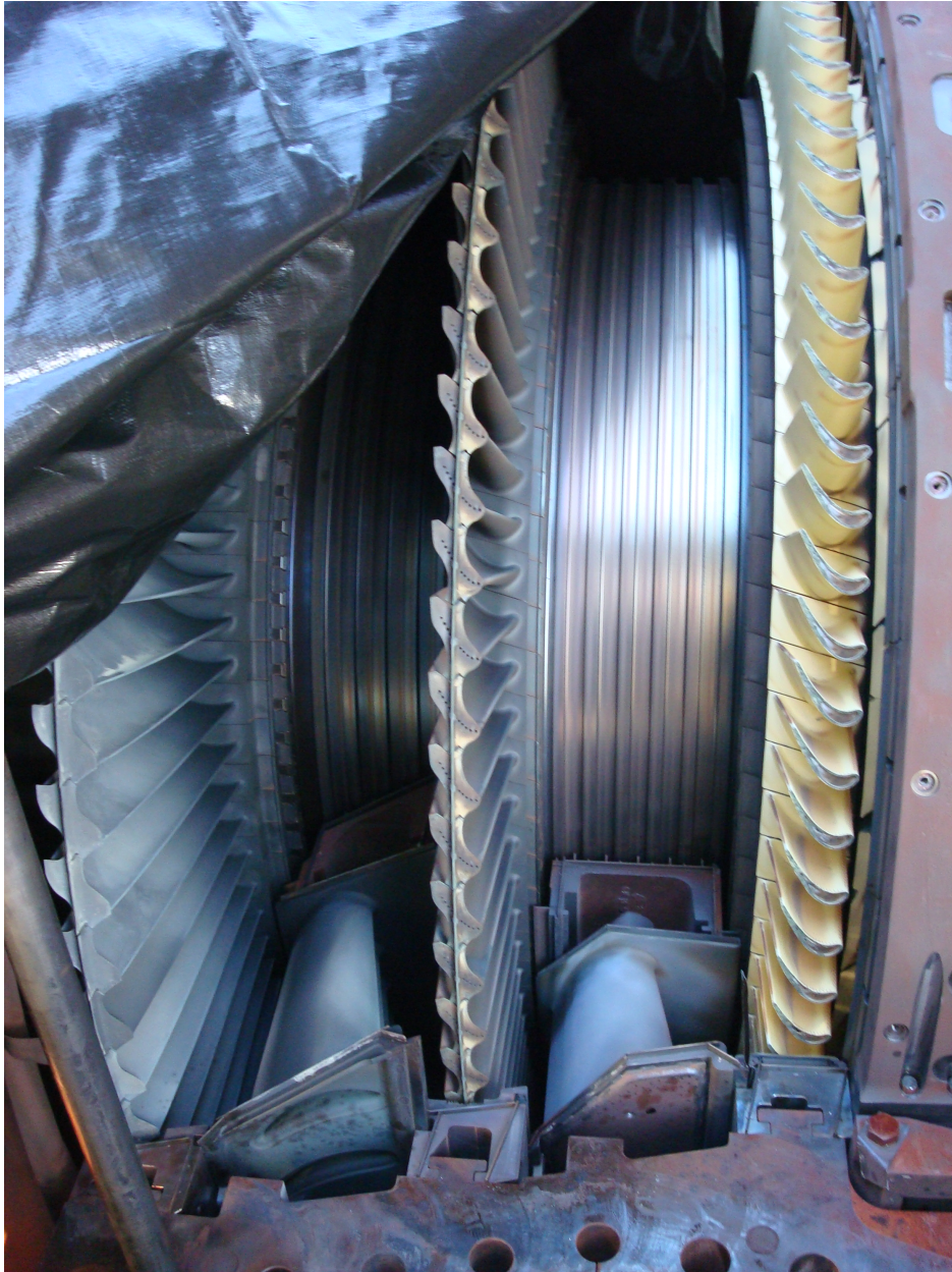
Figure 42. Power plant gas turbine using axially overlapping seal ring configuration
