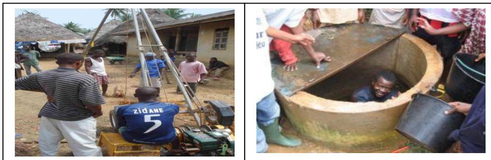
Figure 5. Typical Well Drilling in West Africa Percussion drilling equipment (on left) and hand-dug well (on right)
