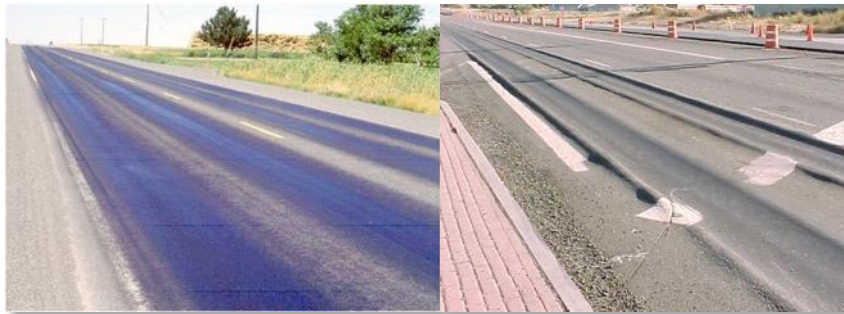
Figure 2- 3 Asphalt Pavement Distresses: (a) Bleeding, (b) rutting (LDOT, Pavement Interactive)
