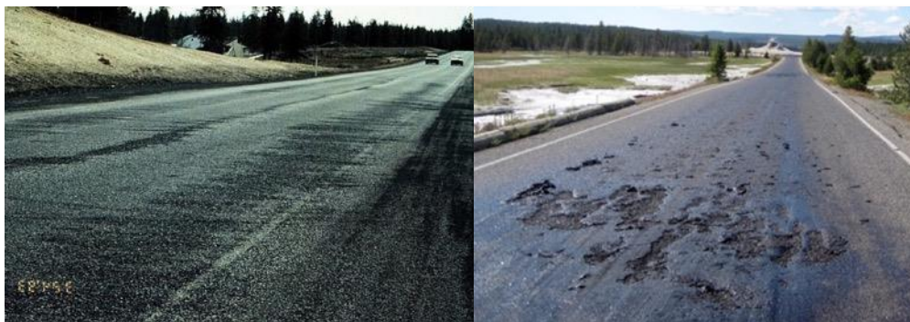
Figure 2- 5 Asphalt Pavement Distresses: Raveling (Pavement Interactive, Yellowstone Park)
