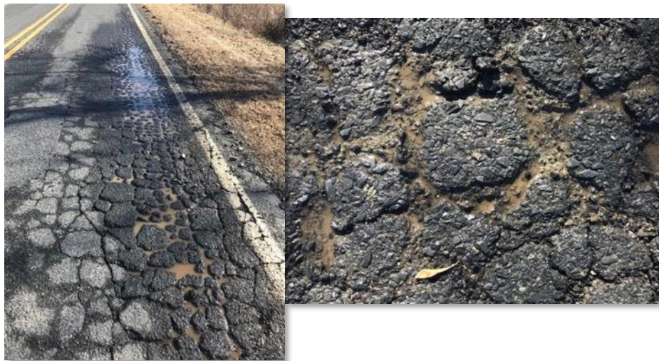
Figure 2- 4 Asphalt Pavement Distresses: Cracking
