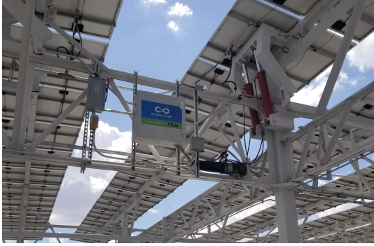
Figure 2.6: Electrical and Mechanical Components of PV Modules at ASU Apache Parking Structure.
