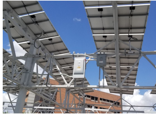
Figure 2.7: Electrical Components of PV Modules at ASU Apache Parking Structure.
