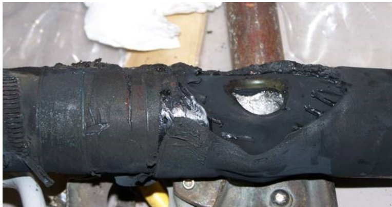
Figure 12.2: Cable Failure In Salt River Project.
