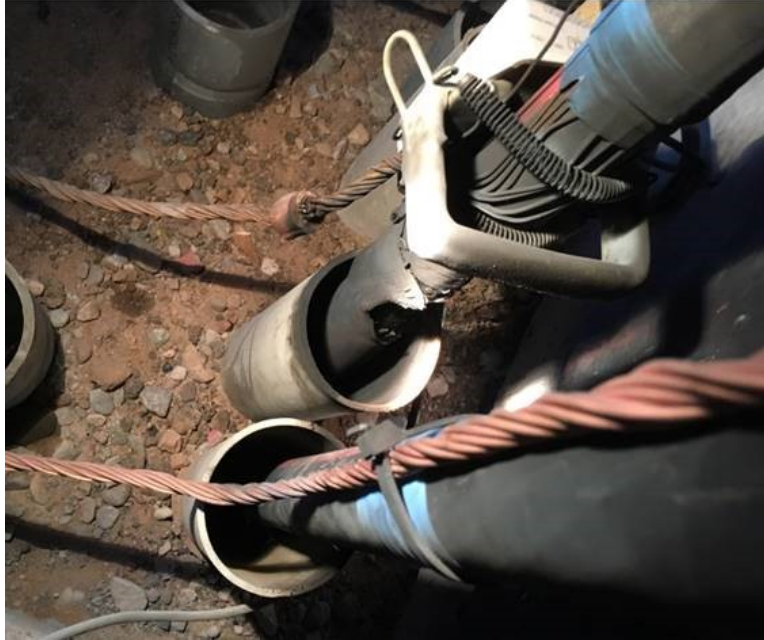
Figure 12.1: Cable Failure For Underground System.
