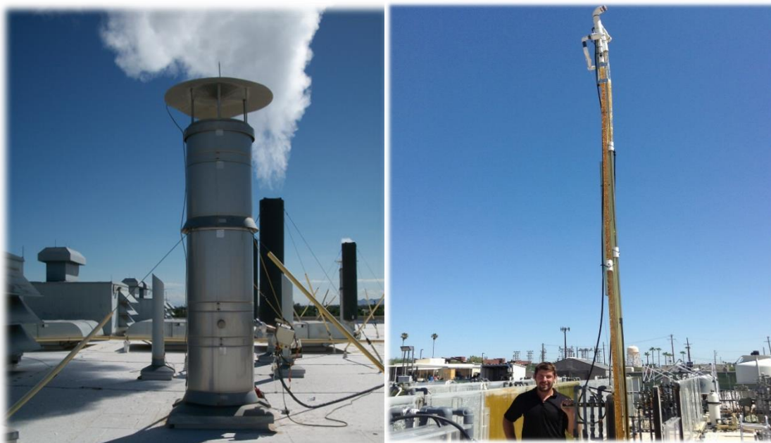
Figure 3. 11: Flue gas stack with sampling port at local semiconductor wafer fabrication plant.
