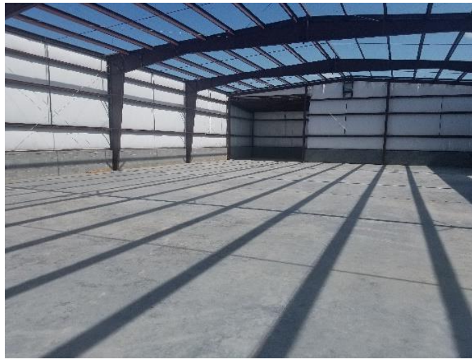
Picture 3.1: Inside Building - Cottonwood, AZ
