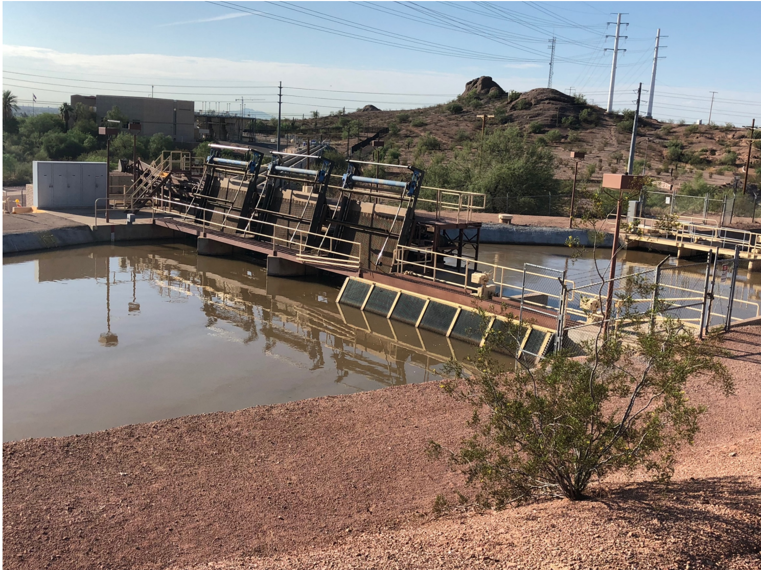
Figure 1-6 SCADA Enabled WSCS Gates Tempe, AZ
