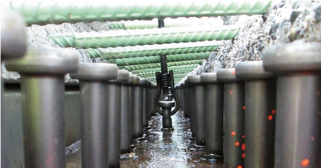
Figure 89. Longitudinal connection detail above first interior girder line with shear studs stopping below the bottom mat of rebar [57].
