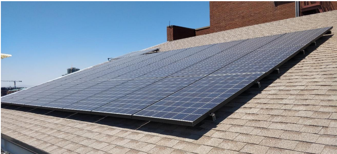
Figure 2.3 Solar panels at the roof of ERC.
