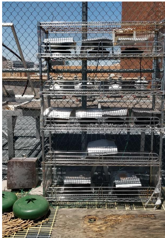
Figure 2.10 The bigger load bank with 10 steps of 880 W each.
