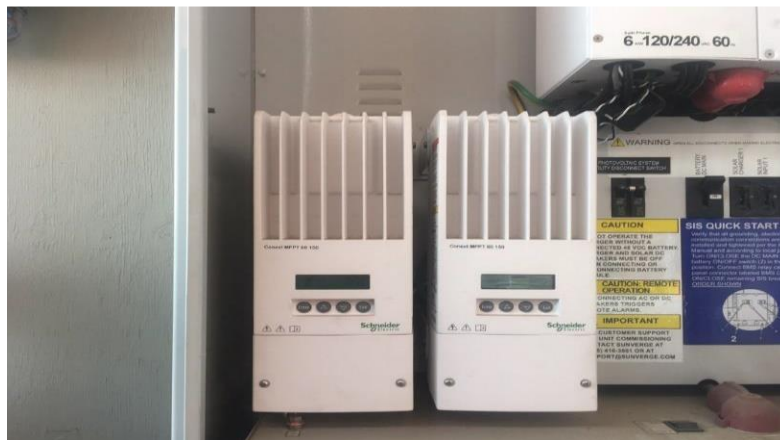
Figure 2.4 The Sunverge MPPT charge controllers.
