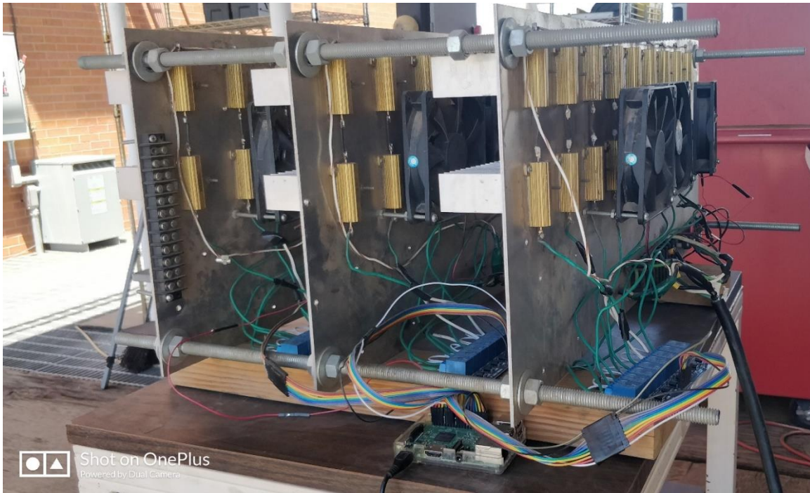
Figure 2.9 The smaller load bank with 29 sets of 72 W steps.
