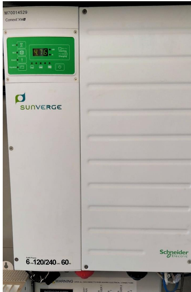
Figure 2.6 The Sunverge inverter
