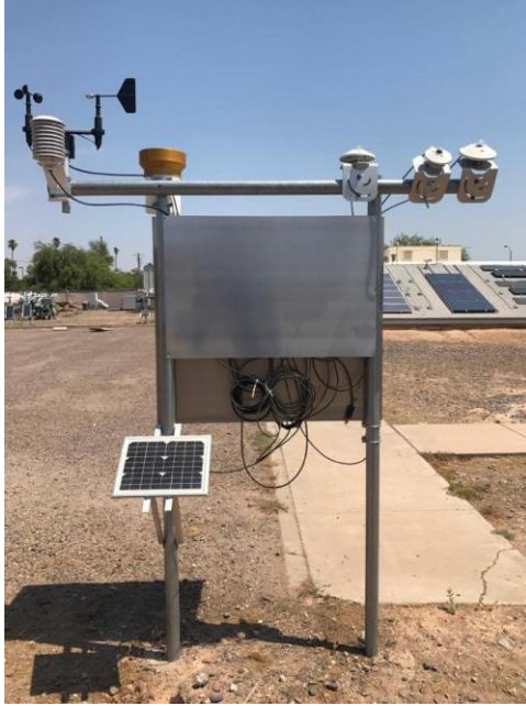
Figure 21 Front view of weather station in the field
