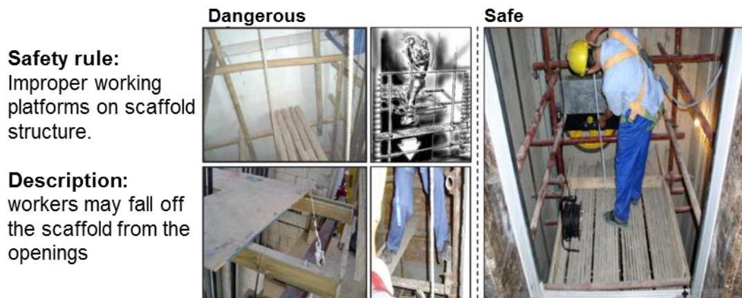
Figure 18. Training Materials of a Safety Rule "Improper Working Platforms on Scaffold Structure."
