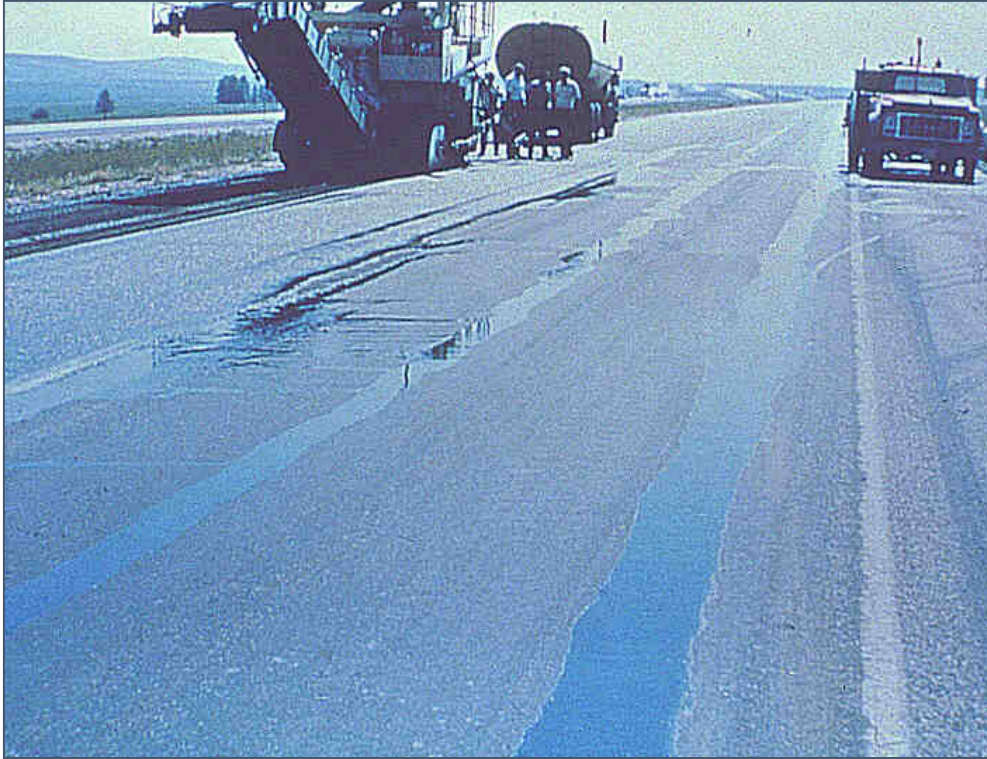
Figure 2. 3 An example of pavement rutting with water accumulation
