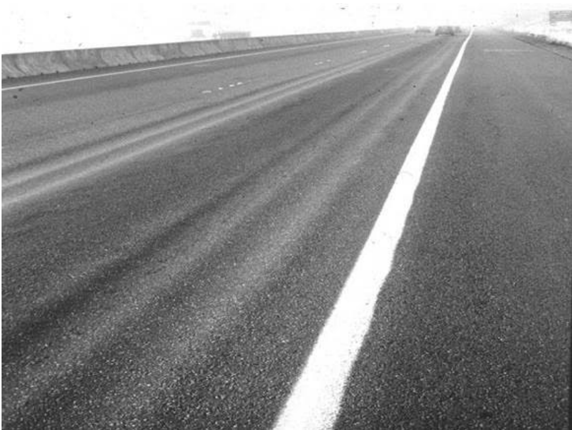
Figure 1.3 Example of pavement rutting
