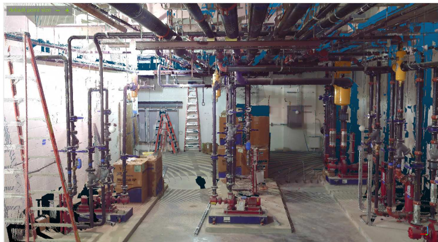
Inside View of the 3D Laser Scanning Data of the Mechanical Room
