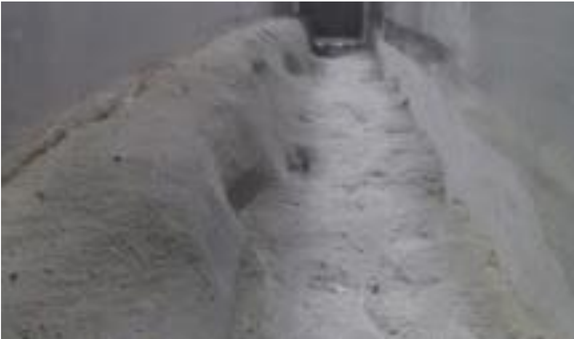
Figure 47: High roughness bed form half-way through manual carving away of outer channel banks.
