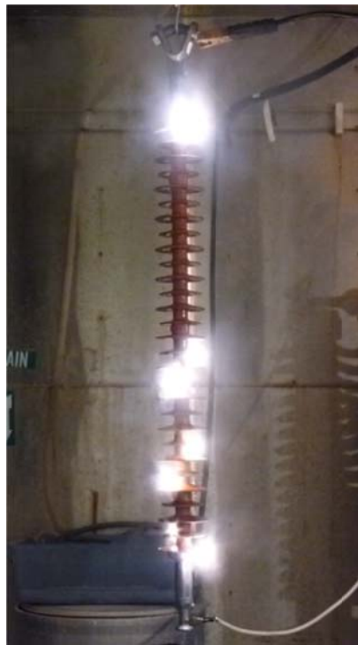
Figure 28. Laboratorial Testing on the Contaminated Insulator Illustrating Arc Jumping Sheds. Bottom Electrode is HV Electrode and Top Electrode is Ground Electrode.
