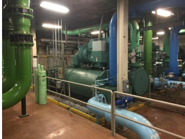
Figure 6: A Chiller from ASU's Central Plant
