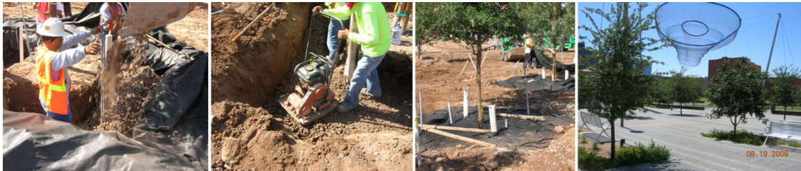
Fig. 2. From Left to Right Installation of Structural Soil and Growth of Trees in 2009 at Civic Space Park in Phoenix, AZ USA.
