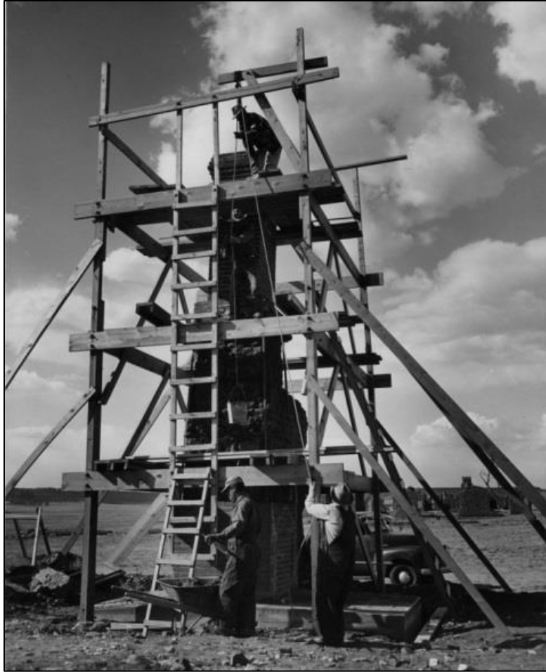
Figure 34: Stabilization of Officer's Quarters, c.1960 (Source: Fort Union National Monument Photo Files)
