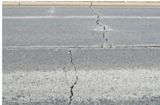
Figure 4: Example of Transverse Cracking in Rigid Pavement
