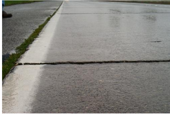
Figure 5: Faulting in Rigid Pavement
