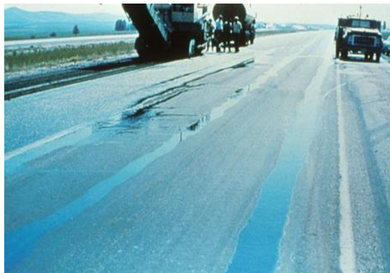
Figure 3: Examples of Rutting Distress in Asphalt Pavement.
