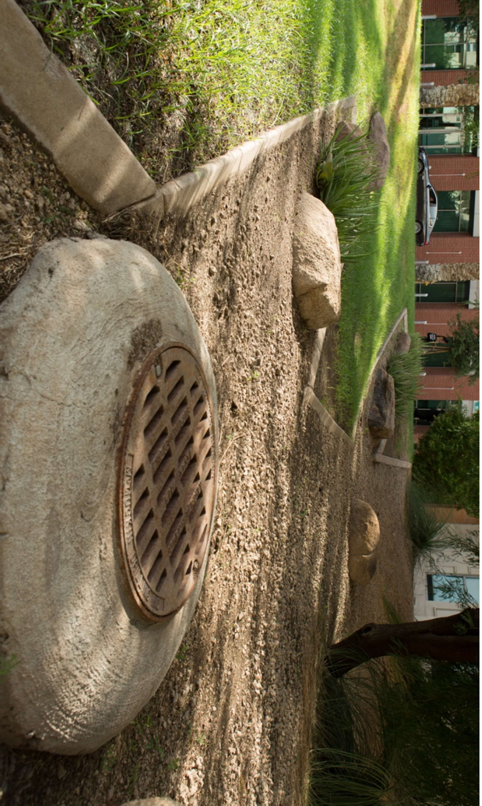
Figure 10. Inlet to a Dry Well Located in the Bioretention Basin Shown in Figure 5. Photo: Mason Lacy
