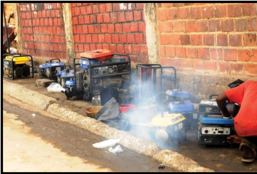
Fig 2.5 Cluster of portable generators outside a local business area. Source: Dada Joseph
