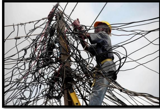
Fig 2.2b Nigeria Power employee works on a tangle of lines in Lagos. Source: Sunday Alamba/Associated Press
