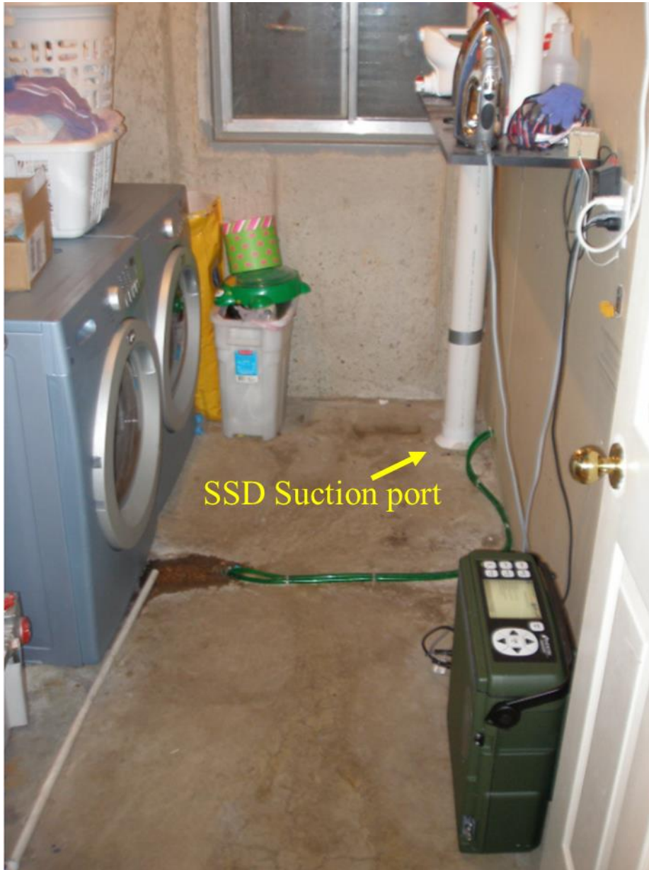
Figure A.10. Photo of sub-slab depressurization system, taken on February 2010.
