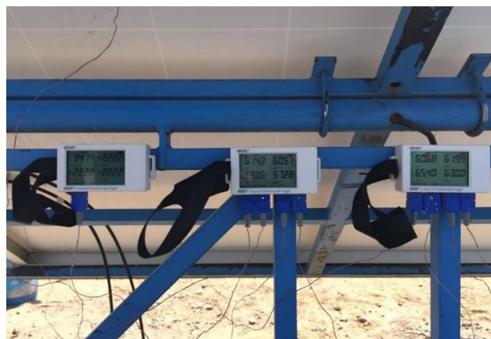
Figure 15. Data logger set-up for short-term monitoring
