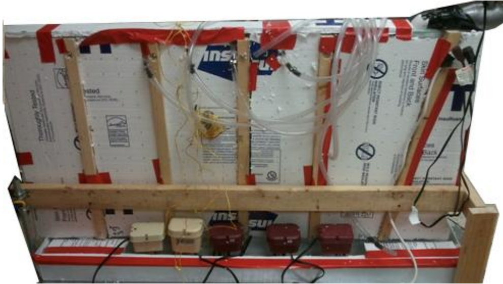
Figure 15. Thermal insulation on the unit and basin to address Challenge 6. The insulation fits between the wooden beams, and the wooden beams also act as insulation.
