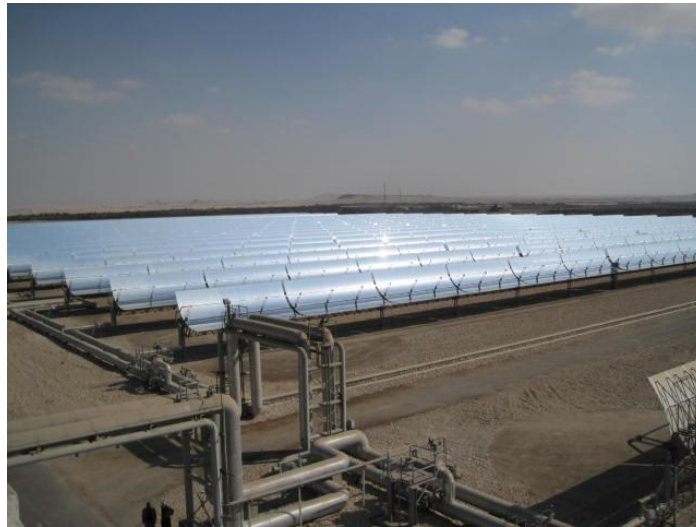
Figure 5. Kuraymat CSP Trough Field Added to a Natural Gas Plant, 2010 Near Cairo, Egypt. Photo by Author.
