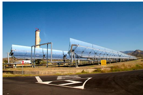
Figure 19. DISS Parabolic Trough. Source: Plataforma Solar 64
