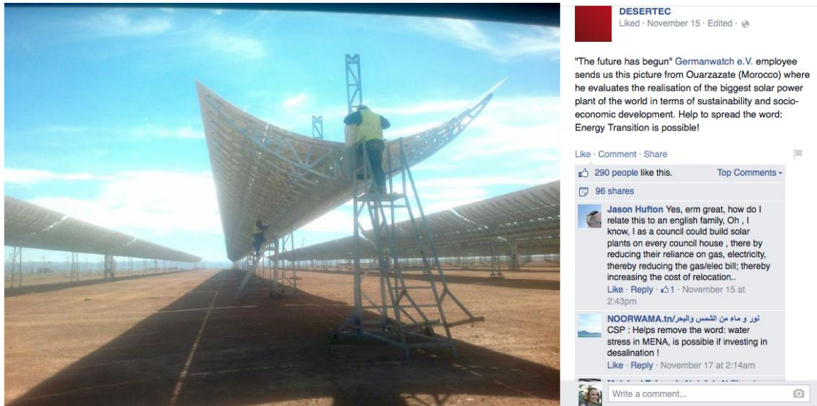
Figure 61. Noor I under Construction on the Desertec Foundation's Facebook Page. Screenshot by Author.
