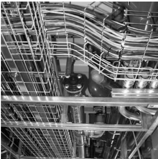
Electrical and gas piping "highway"
