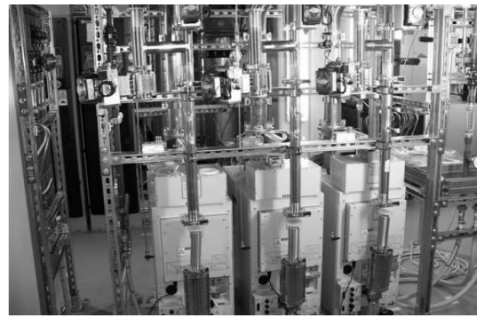
VMB's and distribution racks in sub-fab
