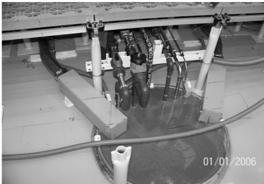
Utilities under the raised metal flooring (RMF) through the pop-out to the sub-fab
