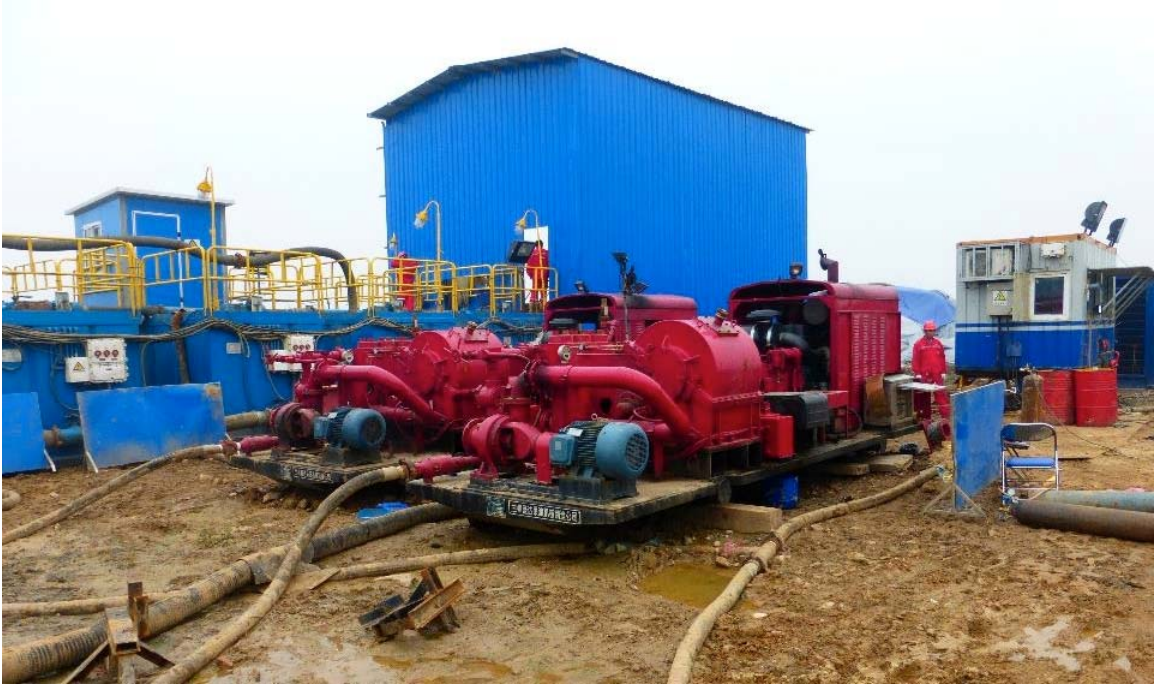
Figure 5.12: Onsite Mud Recycling System
