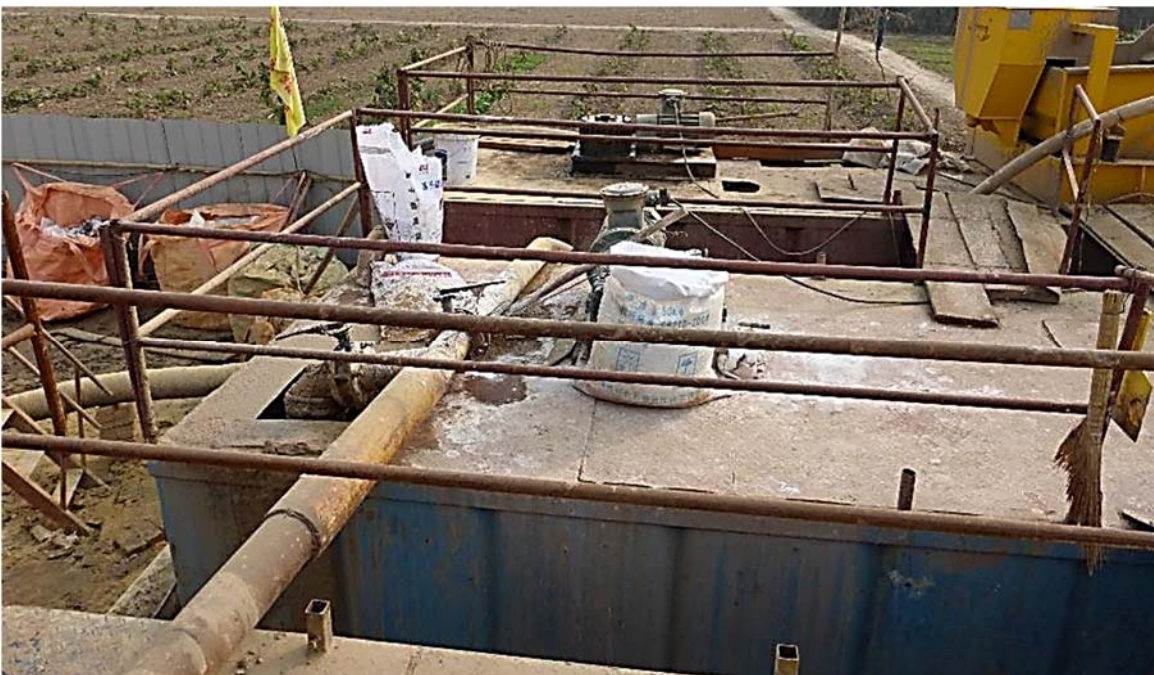
Figure 5.18: Overhead View of Custom Fluid Recycling System
