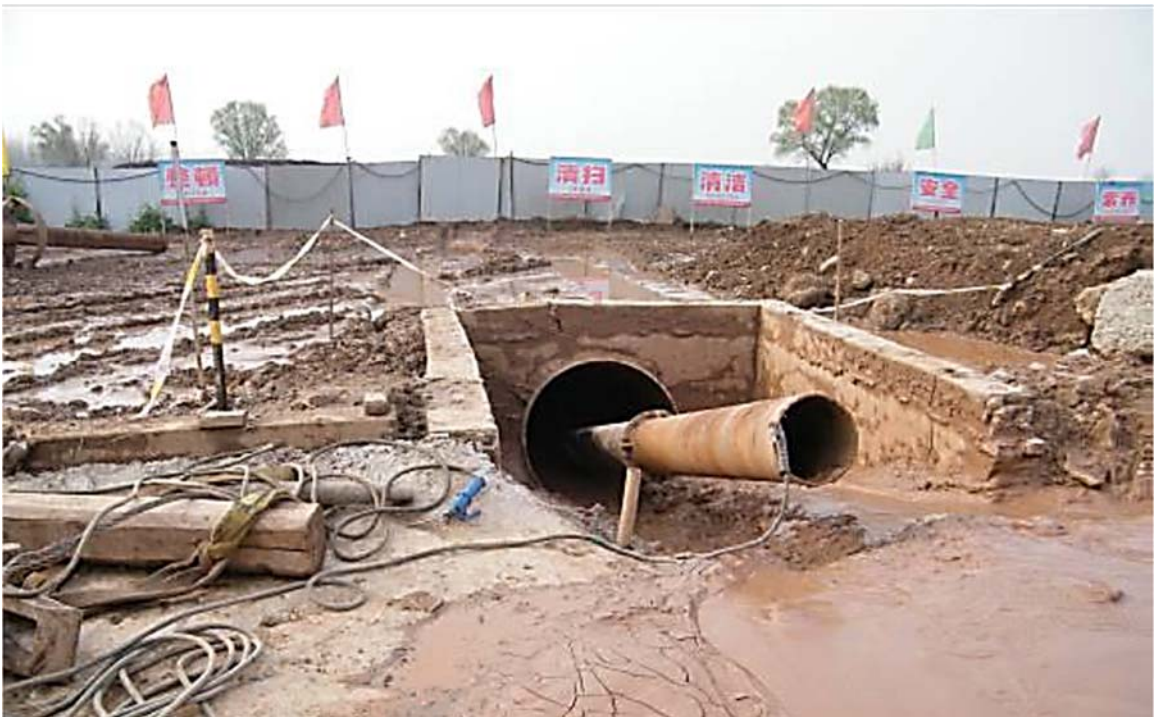
Figure 5.39: Reinstall Center Locator inside Casing on the South Bank (Li et al, 2013)
