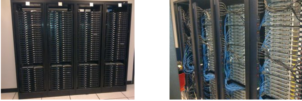
Figure 2.1: BlueCenter, a Small Testbed Data Center at ASU, (a) Front View of Racks, and (b) Back Side of Racks.
