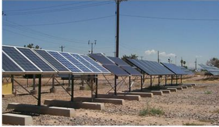
Figure 40: PV Panels in the Field Test
