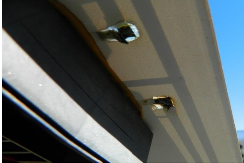
2 Backsheet Burn Due to Solder Bond Failure [1]
