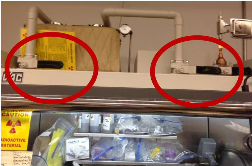
Figure B.9. Blower power switch, blower inlet and output valves locations.
